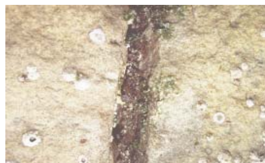
A Crevice in a Seawall
